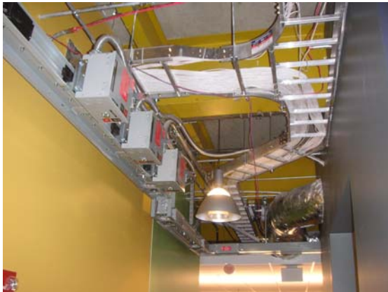
1,200A "Plug & Play" busway & Cable Tray Infrastructure
