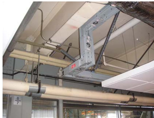
1,200 A Busway distributed up and around drop clouds & Infrastructure
