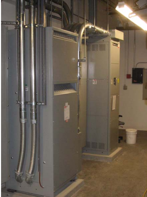
300 kVA harmonics mitigating transformer (left) routed with pipe and wire to a 1,200 A disconnect and transition to busway (right)
